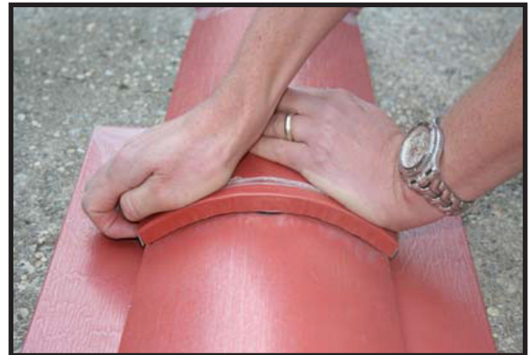
Tile installed properly will fit tight on to lower tiles, do not trim off edges of tile flange.
