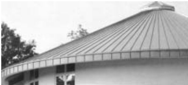
FIG. 2: TAPERED TEE-PANELS FORMED ON THE SL-24 ARE USED ON CONICAL OR ROUNDED CORNER ROOFS
