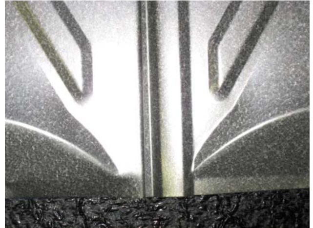
4. It may be required to field adjust the lower left of the shingle's male side in the female "S" to keep the top of the shingle aligned with the chalk line note a minimum of 75% of the shingle should be engaged.
