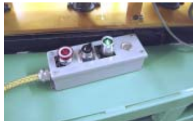
Close Up of Automated Shear Wired Manual Control
